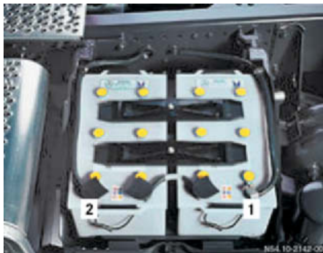
Battery box (1) on driver side (implement carrier)
