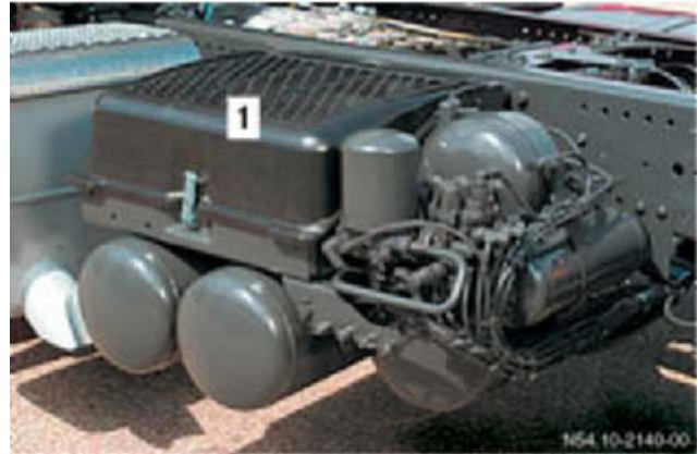
Battery box (1) on driver side (implement carrier)
