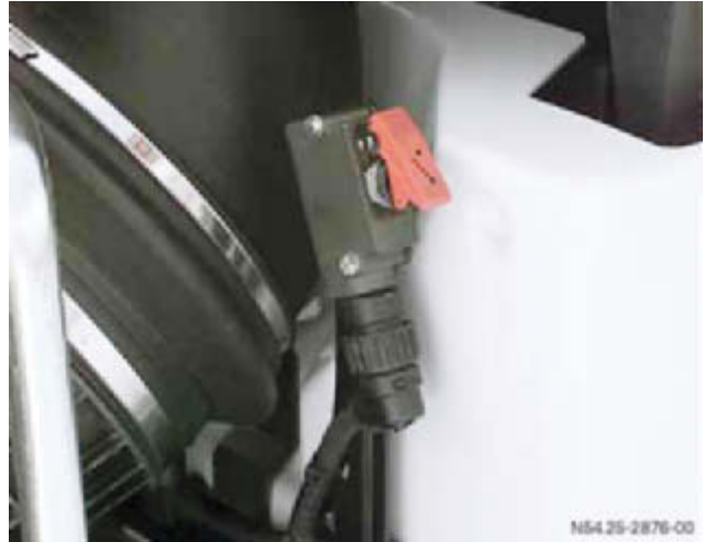
Possible location of EMERGENCY OFF switch on the right behind the cab
