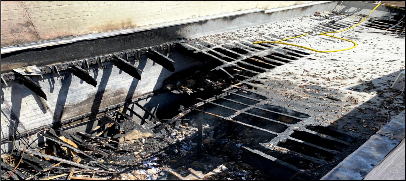
Perspective of roof from Bravo exposure looking back towards the Alpha side
