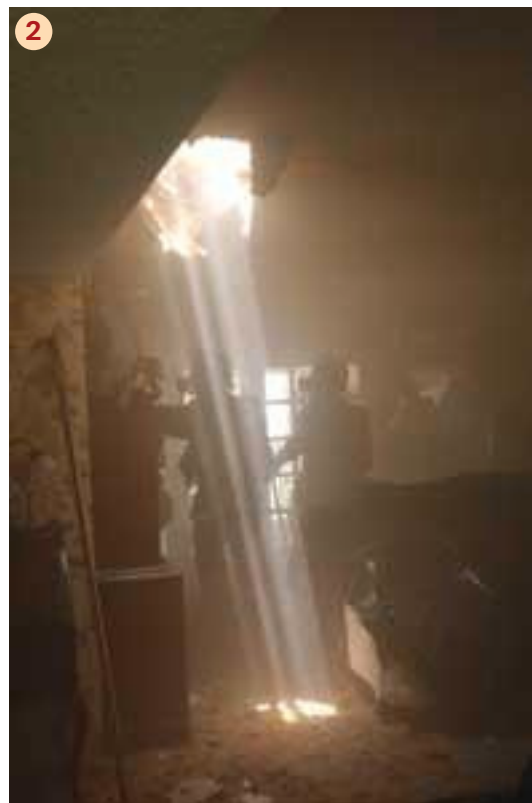
(2) Phoenix Fire Department members wear full PPE, including SCBA, while performing overhaul on a single-story residence.
