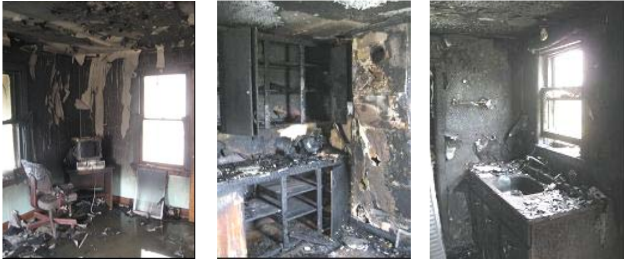
Figure 5-10: Kitchen after the controlled field fire event.
