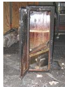
Cabinet (post fire)
